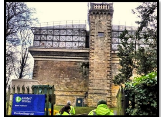
Prenton Water Tower — as work began to occlude the facade of this iconic structure.
